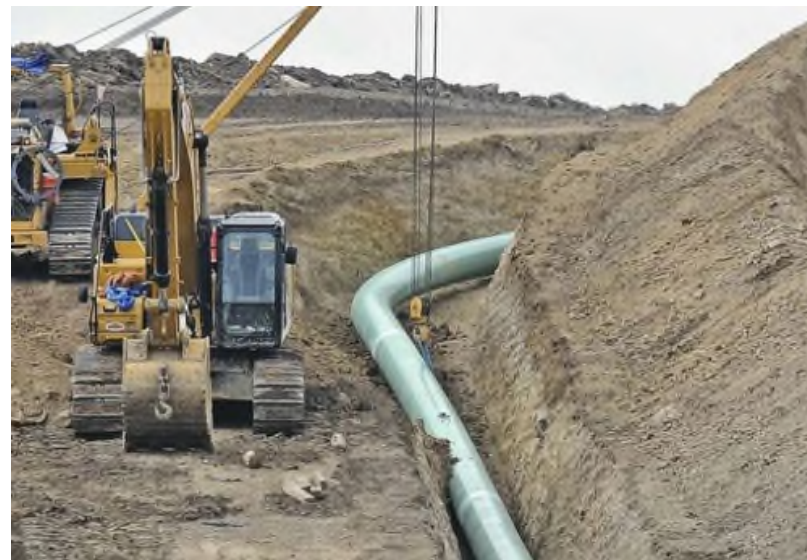
Dakota Access Pipeline: 1,172-mile underground 30" Pipeline from North Dakota Bakken to IL
